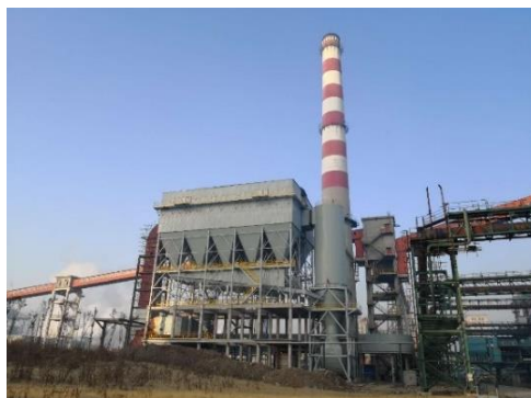
图 3 济南玉泉生物质电厂一体化工程 Fig.3 The integrated removal project of Jinan Yuquan Bio-power Plant
