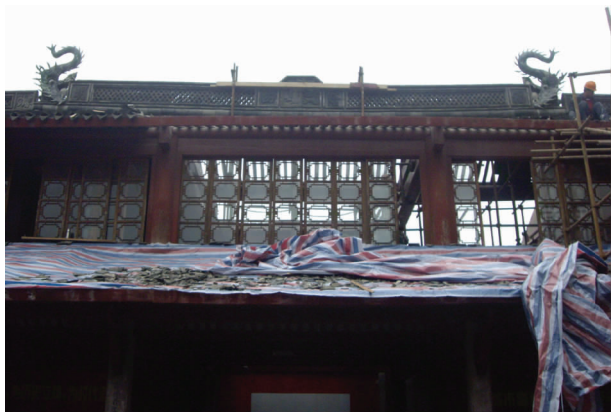
图5 屋面采用了用小木条同屋脊水平方向夹住屋脊 Fig.5 The roof caught by wood battens placed horizontally with the ridge
