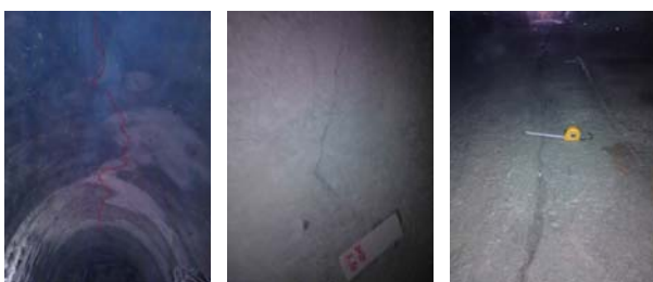
(a) 拱顶裂缝
