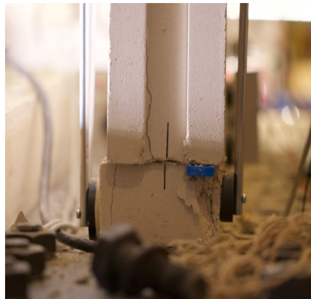
Figure 7. Out-of-plane displacement of element 8 in wide pier 3.
