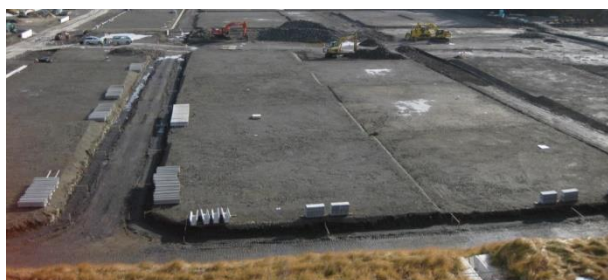
Figure 8. Work area with visible puddles
