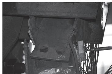
(c) J2处梁腹板螺栓孔受剪变形过大
