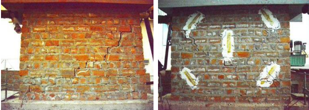
图 20 10-C3-RRBB2 墙体破坏照 Fig.20 10-C3-RRBB2 wall damage photos
