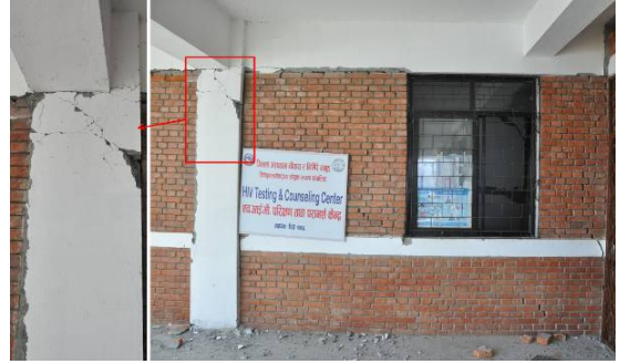
(c) 与小开洞填充墙相邻的柱顶剪切破坏
