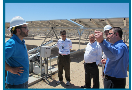
NEPCO delegates tour an APS-owned 17MW solar photovoltaic plant southwest of Phoenix.
