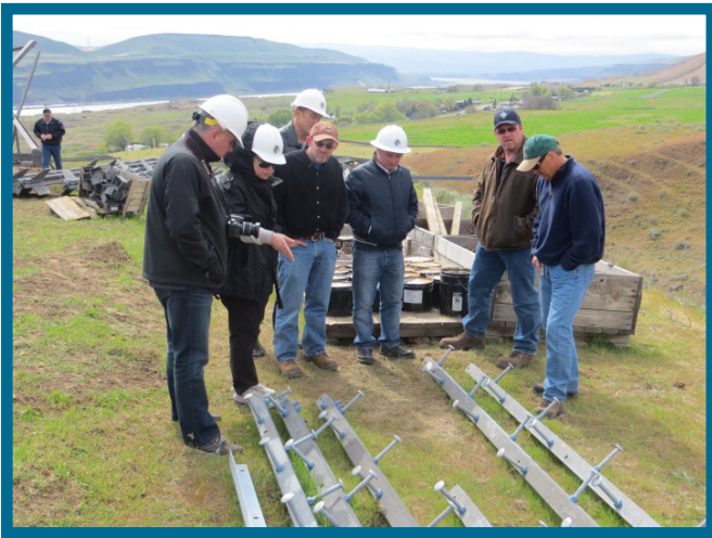
Representatives from the Georgian State Electrosystem tour the Big Eddy-Knight 500kV transmission line construction site near the John Day River Crossing.
