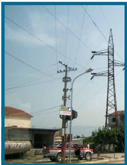
Distribution lines outside Tirana, Albania.
