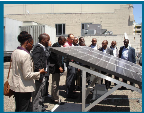
SAPP delegates visit a solar PV rooftop facility at PG&E's Pacific Energy Center.
