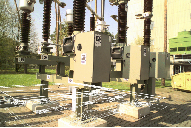
Figure 5: Superimposition of an image and the associated drawing of the scene. Again, the ground plane is not located on the actual ground, but at the top edge of the concrete foundations.
