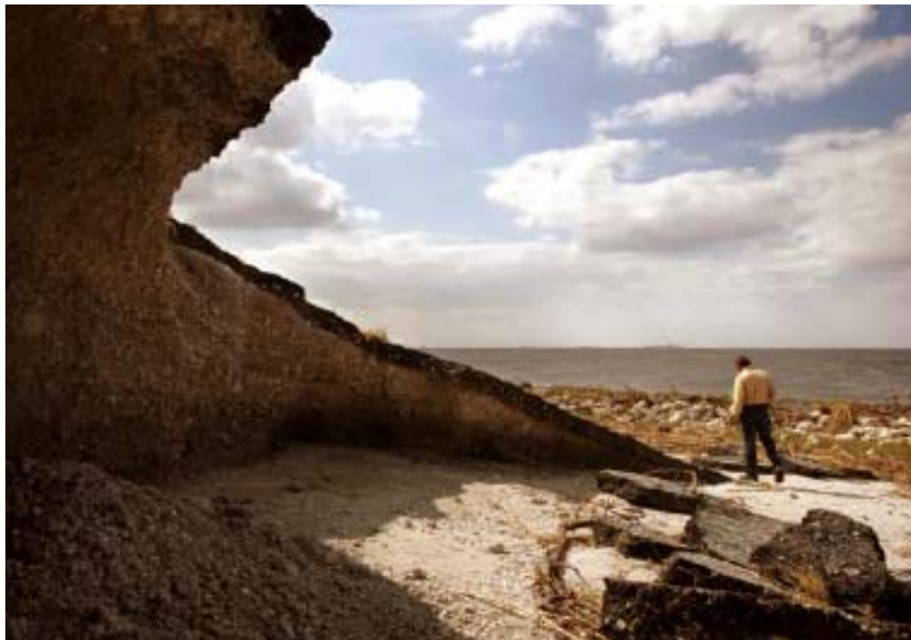
Figure 7. Wave erosion damage to the Herbert Hoover Dike of Lake Okeechobee from Hurricane Wilma (Bromwell et al., 2006).
