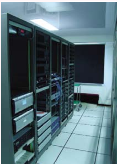
机房 Computer room
