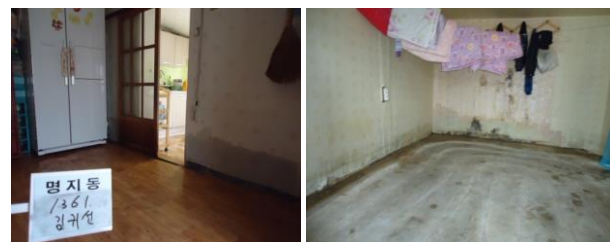
Figure 3. Flooded house' wall and floor
