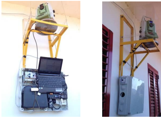
Figure 7. The total station and the control panel
