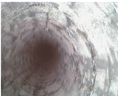
(a) 顶板 1740mm 纵向裂隙 (a) Longitudinal fissure roof 1740mm
