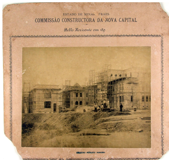
Figure 3.8 “Building of the Secretary of Education under construction.” Workers can be seen in the foreground of the photograph. Raimundo Alves Pinto, photographer. 7 August 1894–November 1896. Photo courtesy of the Arquivo Público Mineiro.
