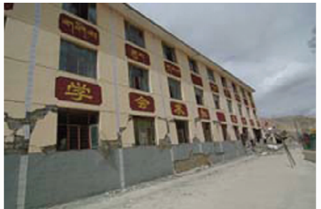
图 10 宿舍楼窗间墙破坏
