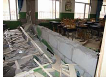
图3 填充墙整片倒塌 Fig.3 Entirety collapse of filled wall
