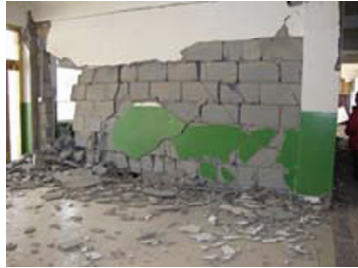
图2 填充墙开裂严重局部倒塌 Fig.2 Severe cracking and local collapse of filled wall
