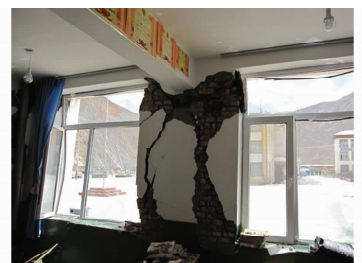
图6 窗间承重墙开裂 Fig.6 Crack of load-bearing wall pier
