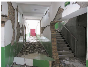
图5 房屋内纵墙局部倒塌 Fig.5 Local collapse of interior longitudinal wall
