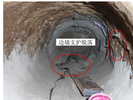
(b) Z = 85 cm 处拱顶、边墙支护开裂、脱落
