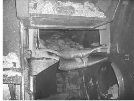
(a) 碴仓出口主筋板冲击挤压破损
