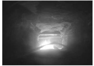
图 2 \lambda = 1.0 时无支护巷道的破坏状态 Fig. 2 Damage status of tunnel in \lambda = 1.0
