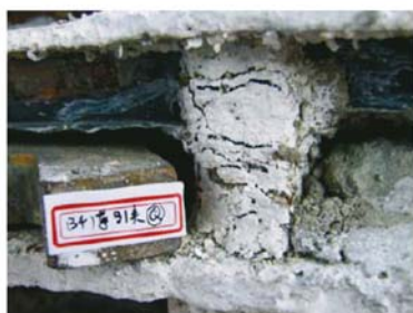
图7 振动台试验中立面收进层柱的破坏 Fig.7 Experimental damages of a column in story with setbacks
