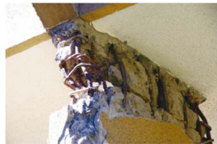
(a) 某剪力墙顶部破坏
