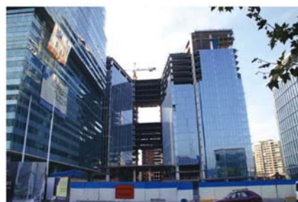
图9 连体高层结构立面照片 [4] Fig.9 Elevation of a multi-tower connected building [4]
