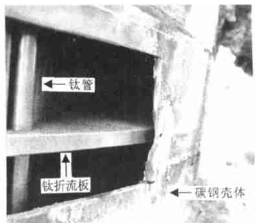
Fig.2 Photo showing corrosion of fluid reflecting plate (From which the samples were cut off) in E-112 condenser
