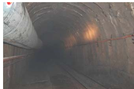
图8 北八运输大巷F2断层核心带巷道维护效果 Fig.8 Maintaining effect of main haulage roadway N8 in fault F2 core zone
