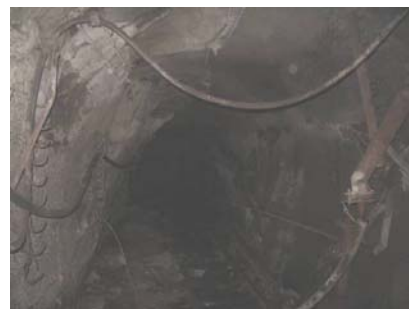
图7 临近区域巷道(北四石门)修复前破坏情况 Fig.7 Destruction of nearby roadway(Shimen N4) before repairing
