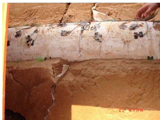
图 10 地裂缝环境下衬砌的破坏 Fig.10 Failure of lining under the environment of ground fissure
