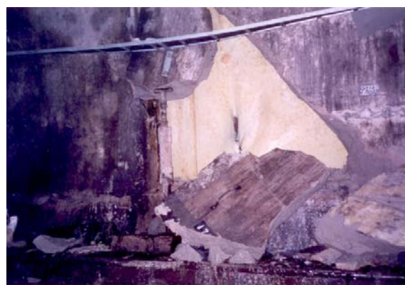
Fig.1 Lining failure due to water pressure [3]
