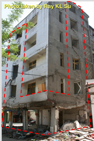
Settlement of columns
