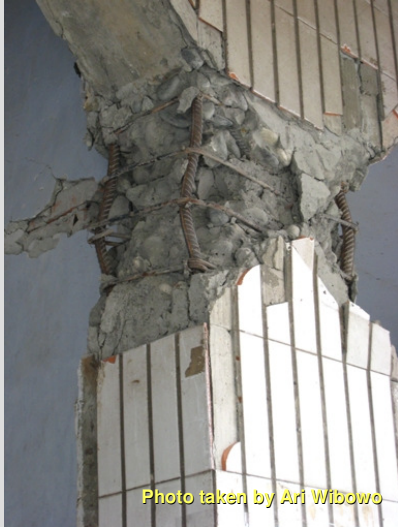
Columns failed in bending and axial load
