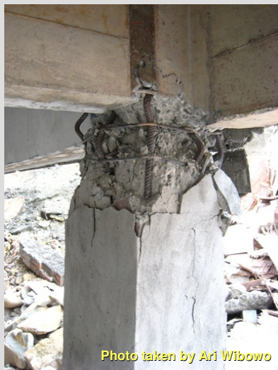
Columns failed in buckling
