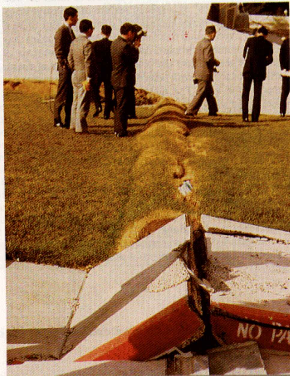
10.16 Disturbed ground and broken sidewalk, Olive View Hospital, San Fernando earthquake of February 9, 1971. [R. Kachadoorian, USGS.]
