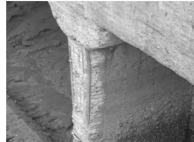
图 9 墩混凝土剥落钢筋暴露 Fig 9 Peeling off of Concrete in Pier and Exposure of Steel
