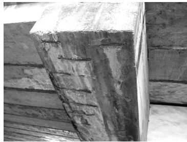
图 2 盖梁混凝土剥落钢筋锈蚀 Fig 2 Corrosion of Steel after Covered Concrete's Peeling off
