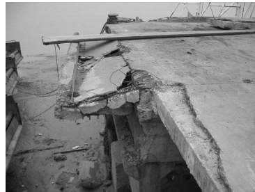
图 8 码头一角超载损坏 Fig 8 Overloading Damage in Wharf
