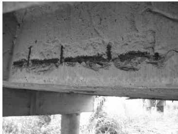
图 7 保护层剥落、主筋锈蚀 Fig 7 Protective Layer Peeling off, Main Steel Corrosion
