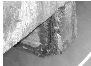
图 12 桩保护层剥落、钢筋锈蚀 Fig 12 Pile Protective Layer Peeling off, Steel Rusty
