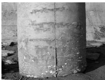
图 13 桥墩横向顺筋锈斑 Fig 13 Lateral Rusty along Steel on Pier
