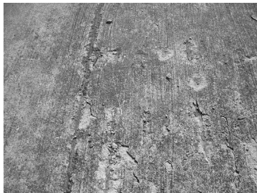
图 10 码头面板混凝土顺筋剥落 Fig 10 Concrete Peeling off Wharf Panel along Steel
