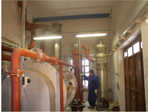
Post burner and off-gas treatment units (2005)
