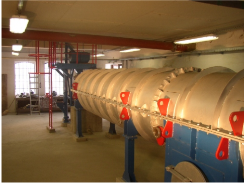
The 3R Anthracite Clean Coal product-like pilot plant main unit: indirectly heated rotary kiln (2005)
