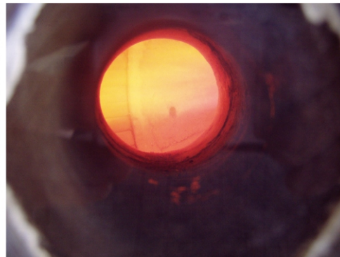
Post burner inner chamber inspection window at operational temperature 850 C (2005)
