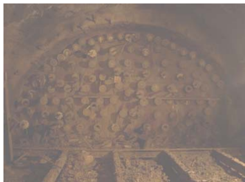
图 6 服务隧洞 F1 风化槽全断面注浆结束后情况 Fig.6 Weathered slot F1 in service tunnel after completion of full-section grouting
