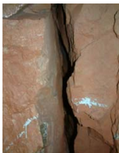
图 7 1 # 平硐拉张裂缝 Fig.7 Patulous cracks for the chamber No.1
