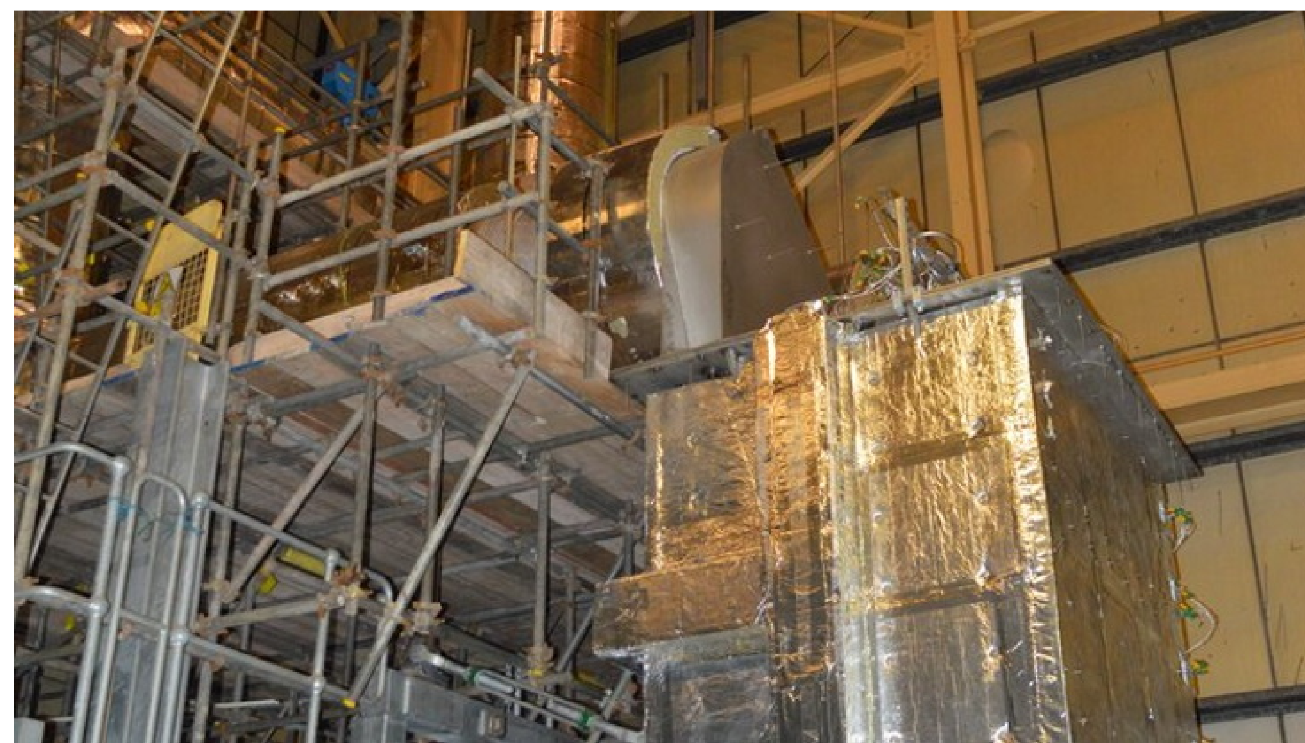
The Passive Heat Removal Facility (Image: Ansaldo Nucleare)
